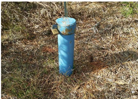
Galvanised steel headworks (GWAN)
