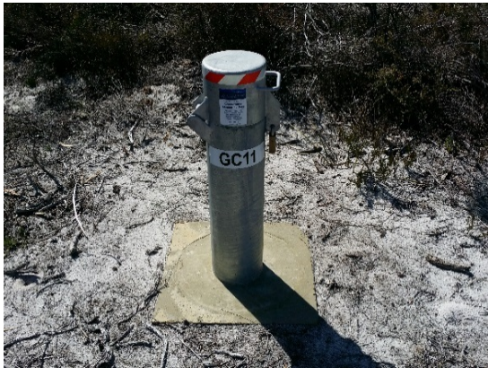
Steel headworks (non-GWAN)
