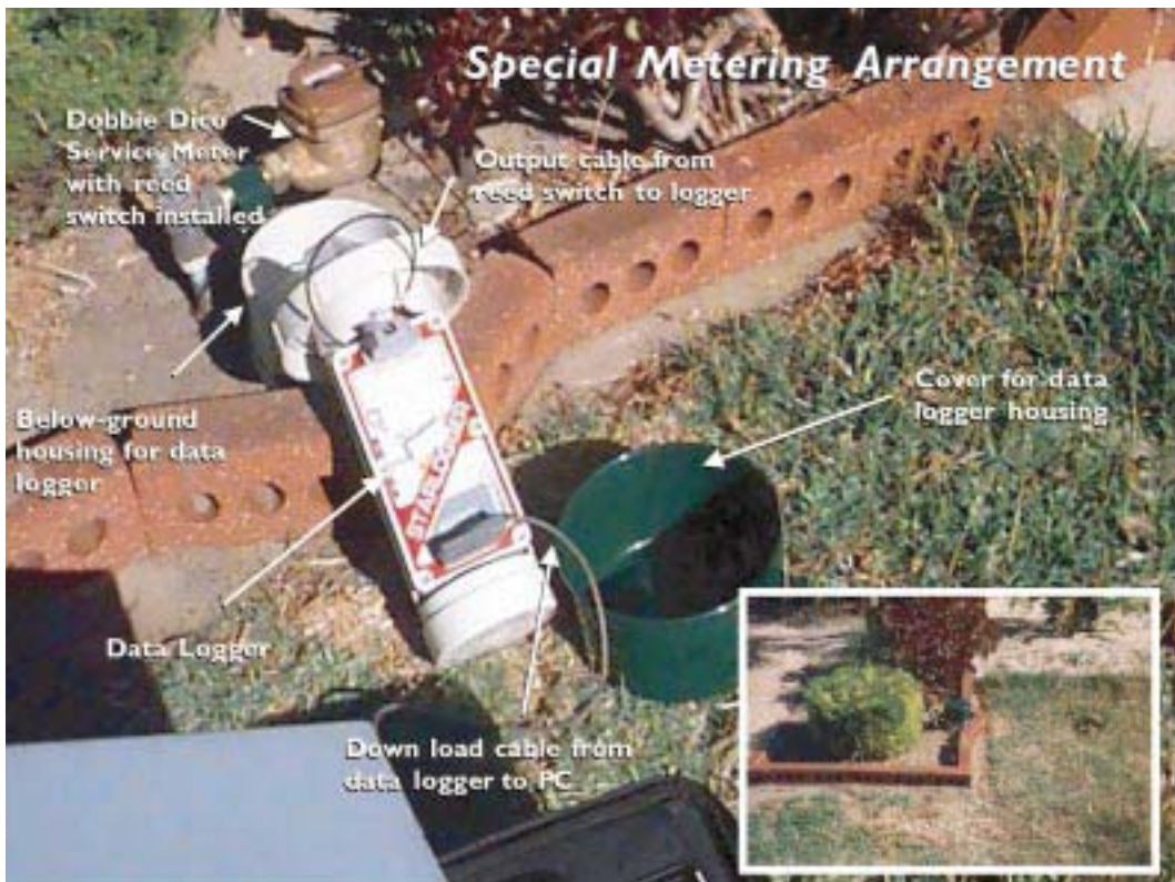
Figure 1.3 ~ 'Smart' Meter Arrangement
