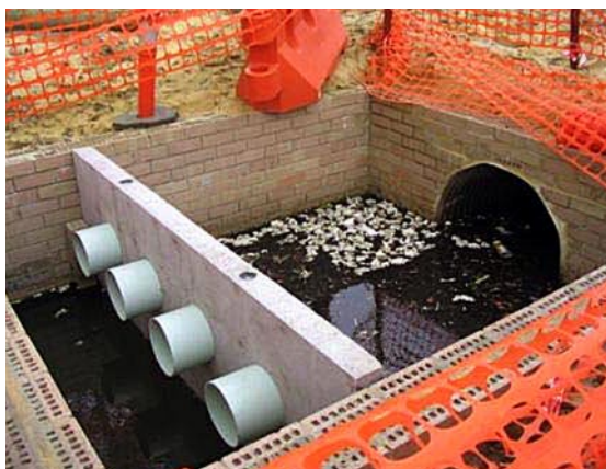
Figure 1. Gross pollutant trap upstream of Liege Street Wetland, Cannington. (Photograph: Department of Water 2004.)
