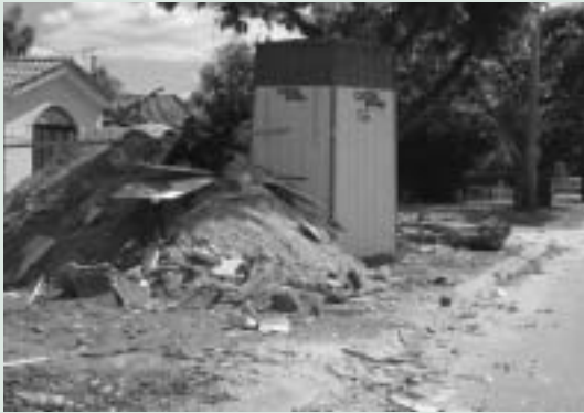
Figure 1. Inadequate waste containment and spillage of waste onto the road. (Photograph: Clean Site, Keep Australia Beautiful Council WA.)
