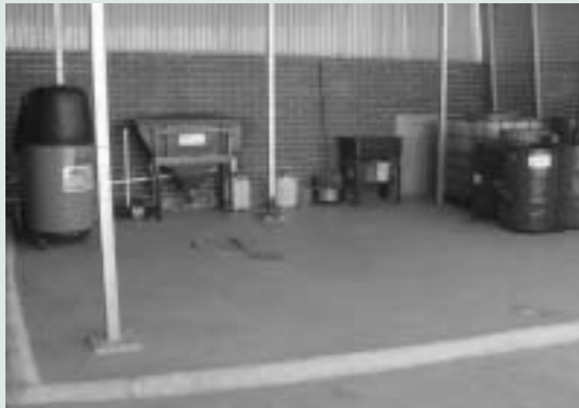
Figure 1. Green Stamp automotive premises, Balcatta. Under-cover, bunded wash-down area, with parts washer, wastewater treatment equipment and drums for recyclable materials. (Photograph: Department of Environment.)
