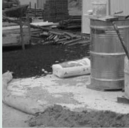
Figure 4. Contained wash area to collect runoff. (Photograph: Clean Site, Keep Australia Beautiful Council WA.)
