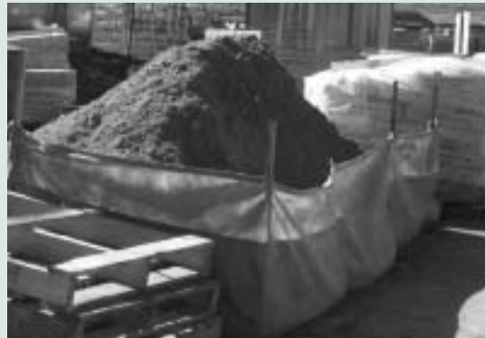
Figure 6. Soil stockpile contained by a sediment fence. (Photograph: Clean Site, Keep Australia Beautiful Council WA.)
