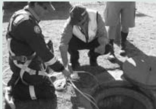
Figure 1. Testing of an industrial site stormwater drain for illicit discharges. (Photograph: Department of Environment.)
