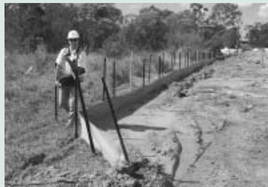
Figure 7. Silt fence for controlling sediment during land development. (Photograph: André Taylor, Ecological Engineering Pty Ltd.)
