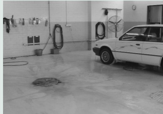
Figure 2. Green Stamp automotive premises, Balcatta. Vehicle wash-down area, with collection drain for wastewater treatment. (Photograph: Department of Environment.)
