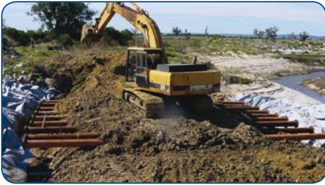
↑ Construction of an offline water reuse storage basin in the Dirk Brook Catchment (Photo: Peel-Harvey Catchment Council)
