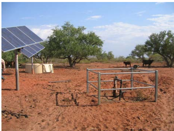
A controlled artesian bore with tank, trough and solar panels which increase efficiency and enable water to be distributed elsewhere on the property.
